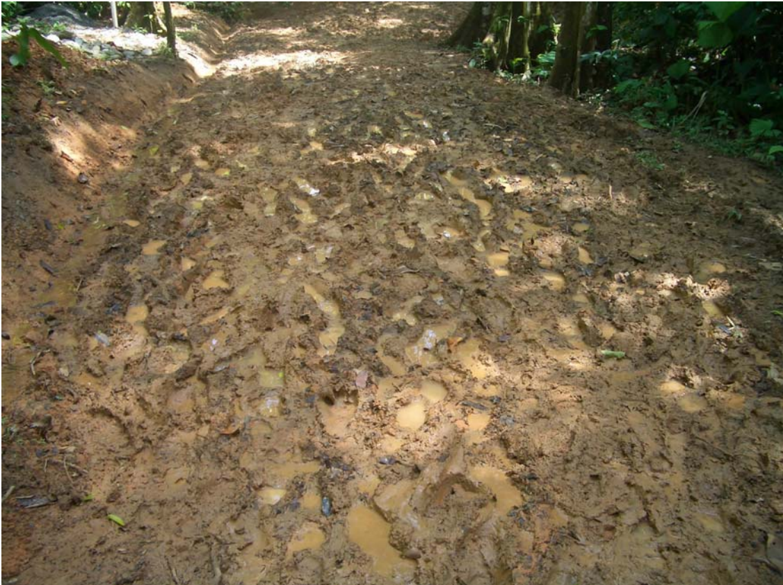
25feb06 - This area is in front of lots 7-9, there is a gradual slope to the left that continually weeps water which runs clean in the ditch to the culvert near the top of the photo. Once it dries up we will compact smooth and either crown or slope. This complete stretch will require 3" GeoWeb for proper support and drainage. Much of the area on the right end of the culvert (top center) is already retained by GeoWeb
