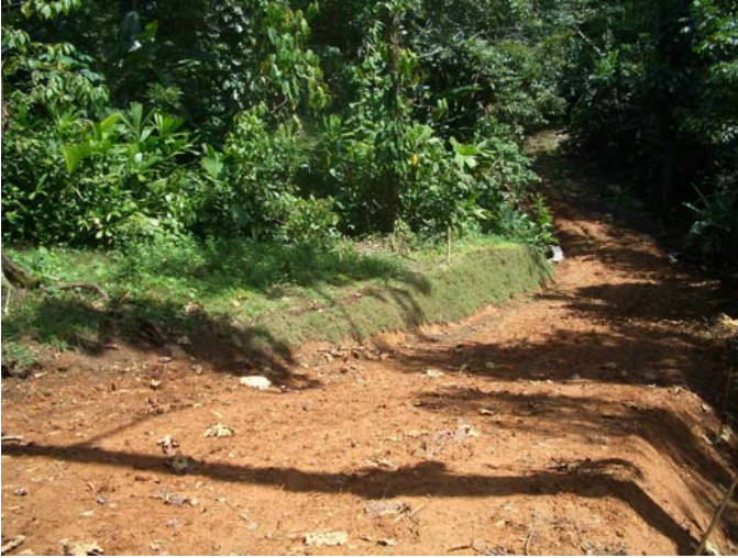
25feb06 – looking east from Lots 2-3, the complete hill was cut out, and sod planted for erosion control
