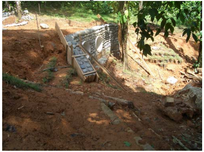
25feb06 – Looking east Culvert Bridge at lots 1-2 w/various erosion control measures, stone outfall construction has also begun
