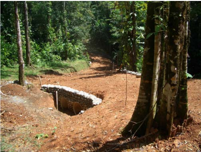
25feb06 - looking East on via Monte lot corner 1-2, Culvert headwall, (Culvert bridge at lots 3-4 is down in center of photo)
