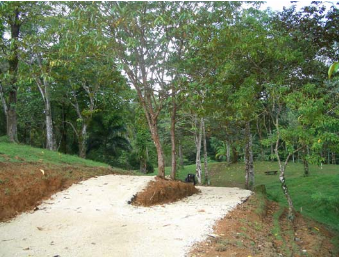
High and low bypass, showing the 4 levels of GeoWeb retaining wall planted with sod, at Lot SB41
