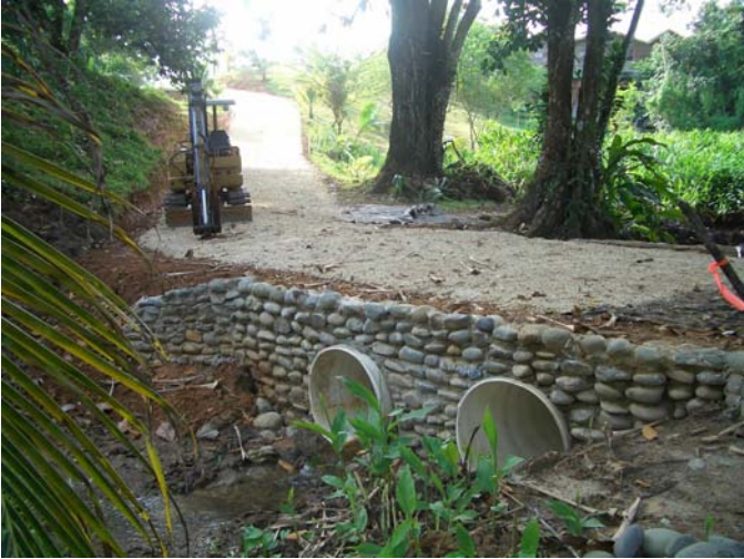
The 1 st Culvert bridge, GeoTextile and base aggregate for the Cart Path at Lots SB16 and SB29
