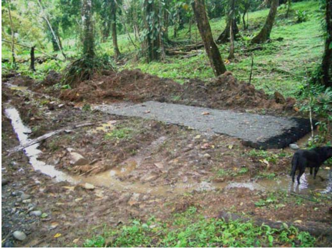
North of SB104 on Via Monte, showing GeoWeb/aggregate Pillow (culvert base) and a diversion ditch during construction
