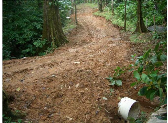
A cut and fill grade on Via Monte at Ridge Lots 8-10. A 3" GeoWeb/aggregate road base will place the full length between the two 18" culverts as a porous road design due to the wetness of the area.
