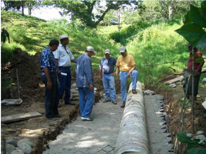
Pillar Construction Engineers inspecting the use of GeoWeb/Compacted aggregate pillows instead of concrete. Two 18" culverts are to be placed here.
