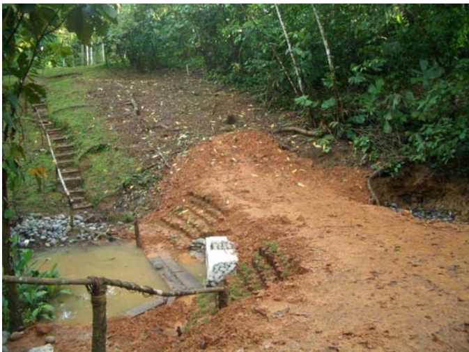
A double 30" culvert bridge spanning what was previously only passable by foot. Again excellent use of GeoWeb was implemented for soil retention.
