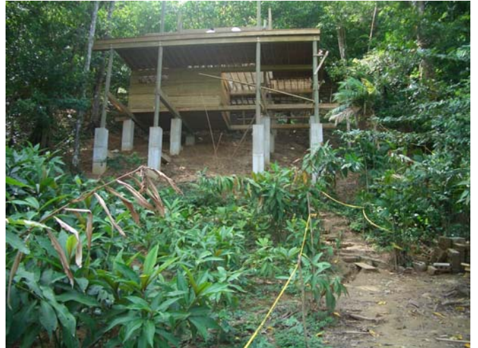
The seismic proofing superstructure of a home under construction perched on a hillside
