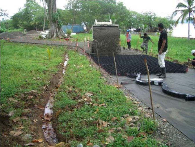
First use of GeoWeb on Solarte. The area is drained and GeoTextile is laid down and then the GeoWeb expanded and staked out prior to filling it with aggregate.
