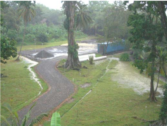
When it rains, it pours in Bocas, but the GeoWeb porous road design holds no water.
